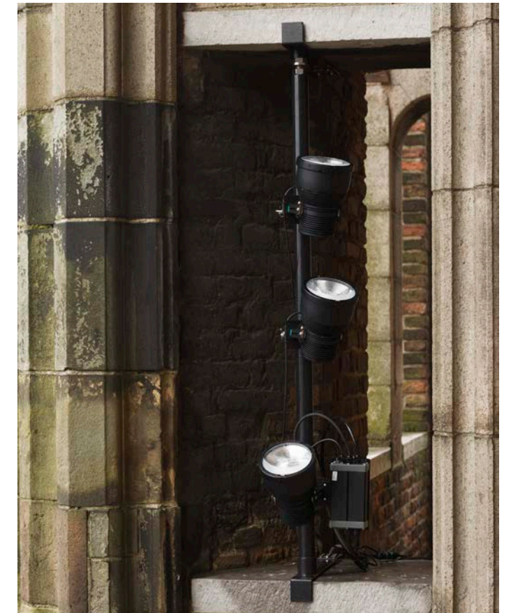
Dom Tower, Utrecht, Lighting fixed in tension
