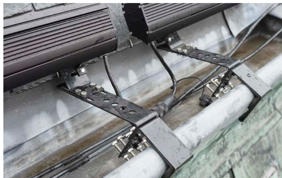
Dom Tower, Utrecht, concealed lighting detail in the architectural fabric.
